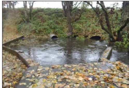
November 23, 2011 flooding at the diversion weir.
