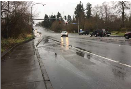
Ponded water at the low point of 44th Avenue W.
