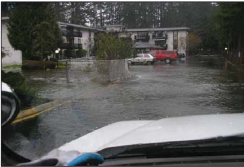
December 3, 2007 overtopping of existing Casa del Rey Culvert.
