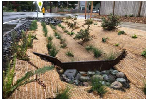
Example bioretention facility.
