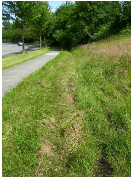
Figure 2. Current condition of drainage ditch along the south side of Alderwood Mall Parkway between 28th Ave and Poplar Way.
