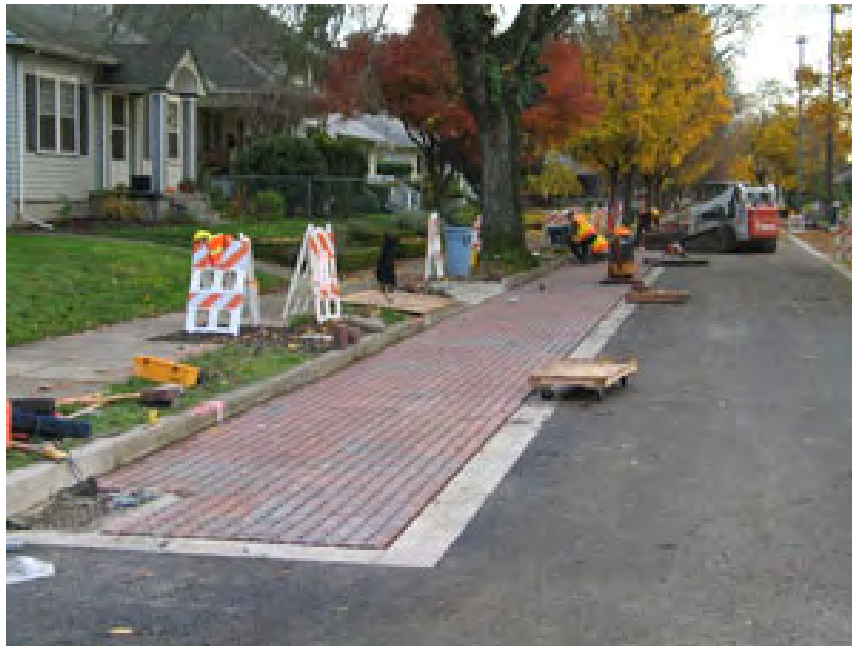
Figure 4-2. Permeable pavement for infiltration of street runoff in a residential neighborhood.
