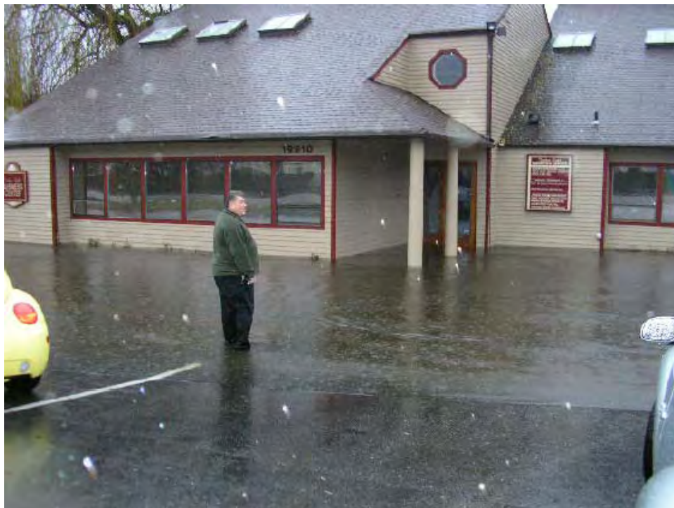
Figure D-6. December 3, 2007 flooding of businesses by Scriber Creek upstream of the intersection of 200th Street SW and 50th Avenue W.
