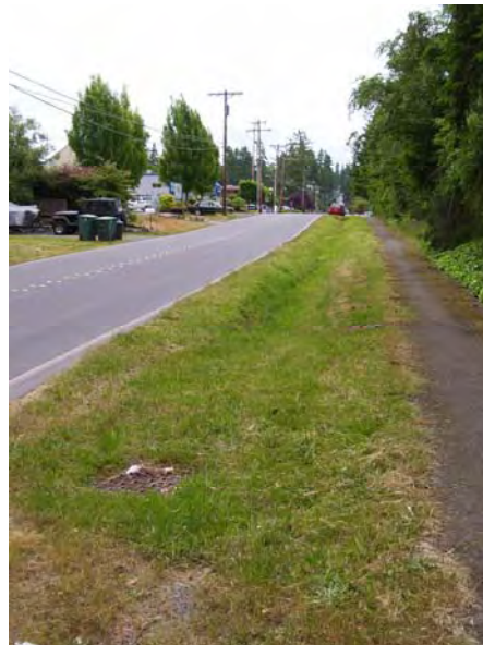
Figure 2. Current condition of unimproved ditch along 180th Ave SW between Hwy. 99 and Scriber Creek.
